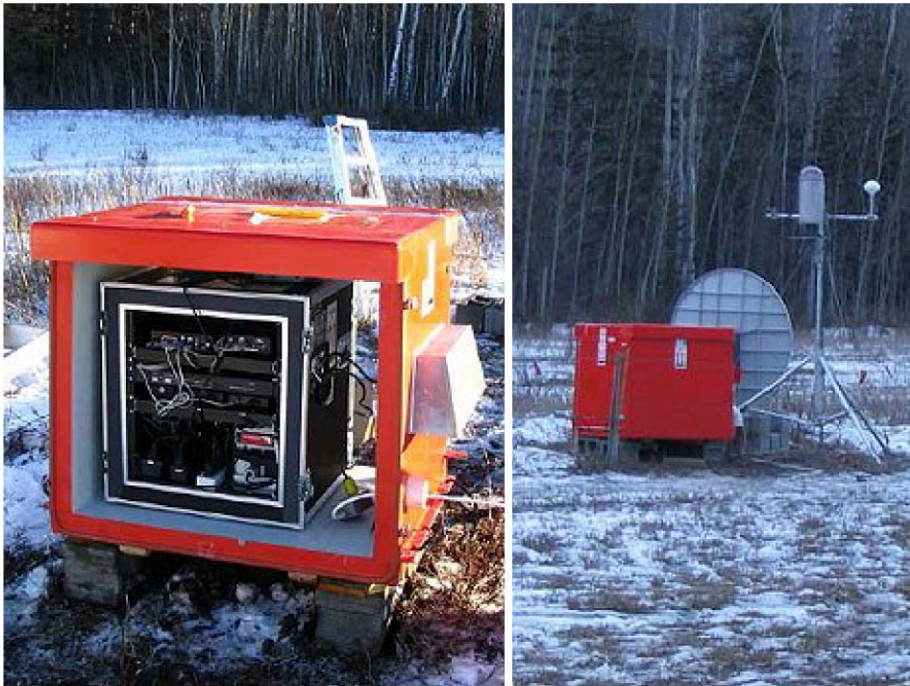
Fig. 8 The GBO site at Ft. Smith during installation. Our enclosure provides a dry and temperate environment for the OSE. When deployed the hut is typically mounted on cinder blocks, or some sort of platform. Tie points on the side rails provide a method to guy down the hut to prevent movement
