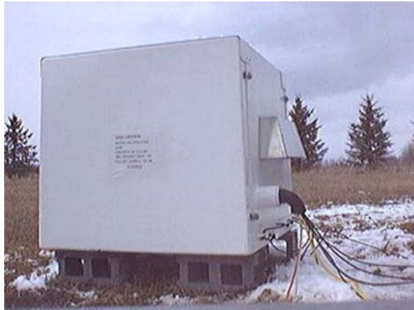
Fig. 3 GBO Prototype at Athabasca University Geophysical Observatory (AUGO). Shown here is the environmental enclosure, designed to house the Observatory Support Electronics, which are inside. On the right side of the enclosure can be seen the shroud covering the solid state air conditioner and the cable access
